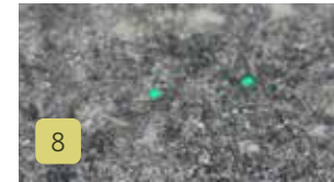
Put the Path Light aside. You should clearly see where the holes need to be placed for your anchors. Drill into each of the marked locations. Make sure you use the appropriate drill bit for the anchor you are using.
