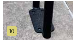
To ensure proper contact, make sure you clean out any debris you made from drilling the holes.
